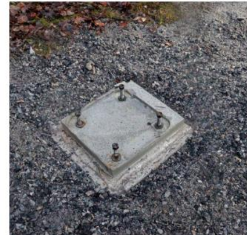
FIGURE 7 SURFACE OF THE GROUT PAD WITH REMOVED COLUMN. CONNECTION WITH THE USE OF HPM® ANCHOR BOLTS
