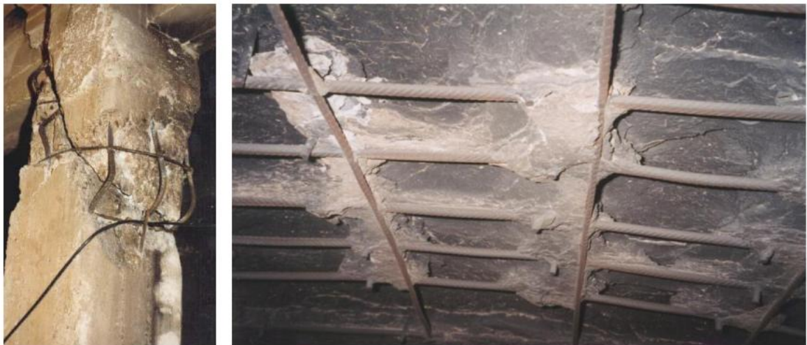
Fig. 4, Some effects of spalling (Innocenzo Mastronardi)
